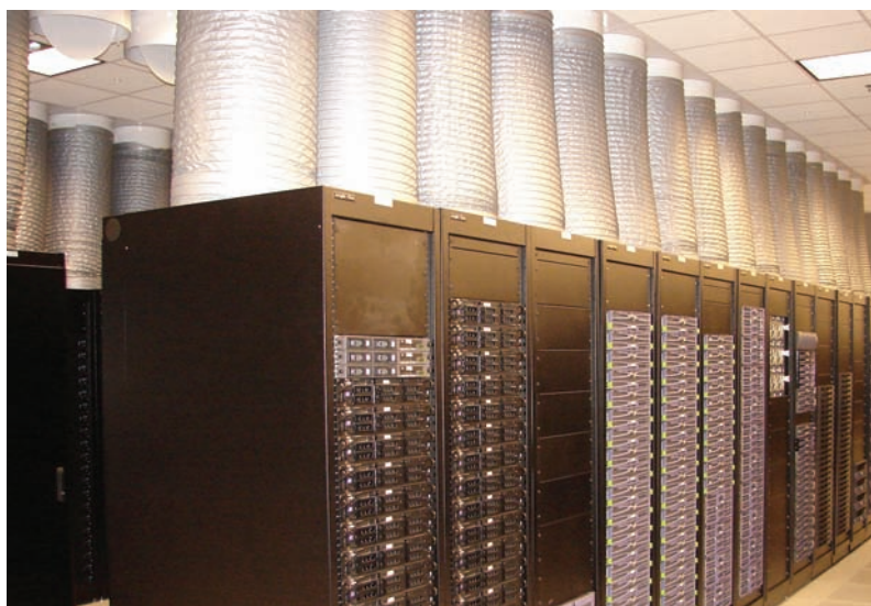
Figure 6: High-density containment systems installed in data center.
